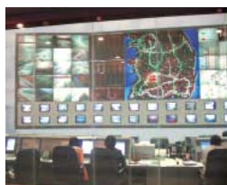
Traffic control center
